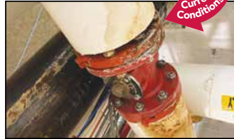
The heating and ventilation system at C-HS is a critical infrastructure need of the building, so much so that the District will attempt to expedite approval from the State Education Department for July '22 construction.
